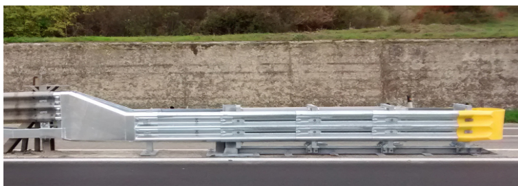
TAU Tube™ P100 installed by a median opening gate
