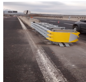
TAU Tube™ P100 installed by a median opening gate
